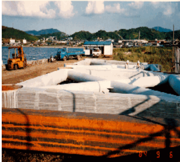
Photo 3 Coating over red rust
