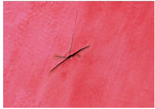
Photo-2 Crack of Fluorine Resin coating
