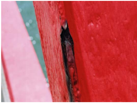
Photo-1 Defective points of Fluorine Resin coating
