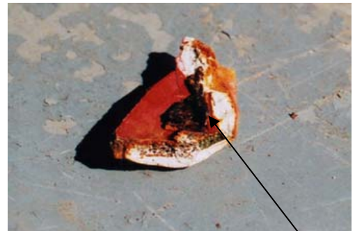
Photo-6 Corrosion where bolt head was removed
