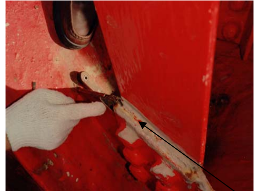
Photo-4 Corrosion of gusset plate edge
